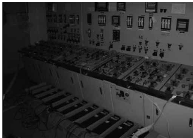
Figure 3. Connected temporary batteries to recover instrumentations in MCR
