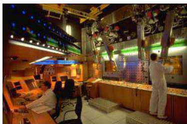
Fig.30: De-storage facility control room
