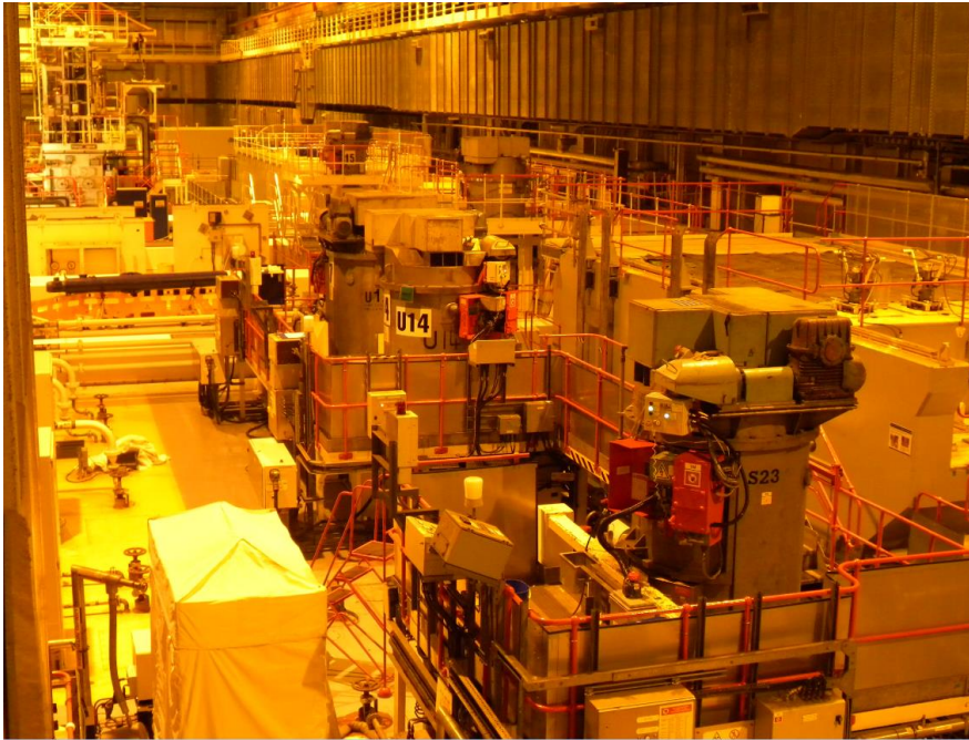
Figure 3 Magnox de-canned fuel Sellafield Packages docked on gamma gates
