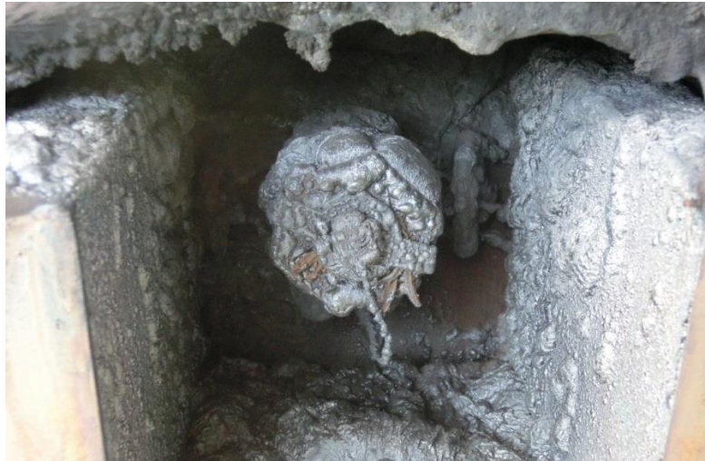
Figure 9: Valve and valve area covered with a black crust (condensation of the decomposition gases of the foam)
