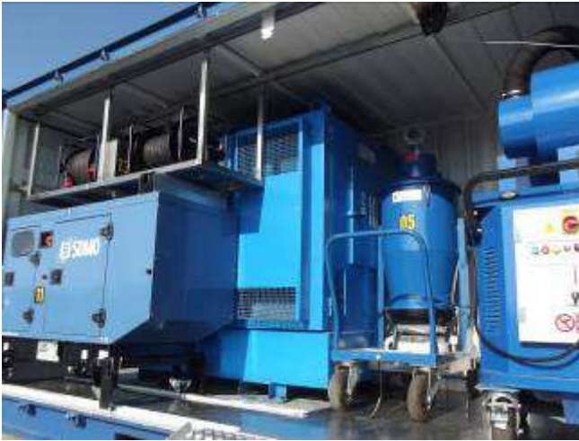
05 - Very High Efficiency Filter 11 - Power Supply In the back - Main Vacuum Pump On the right - Industrial Vacuum Cleaner
