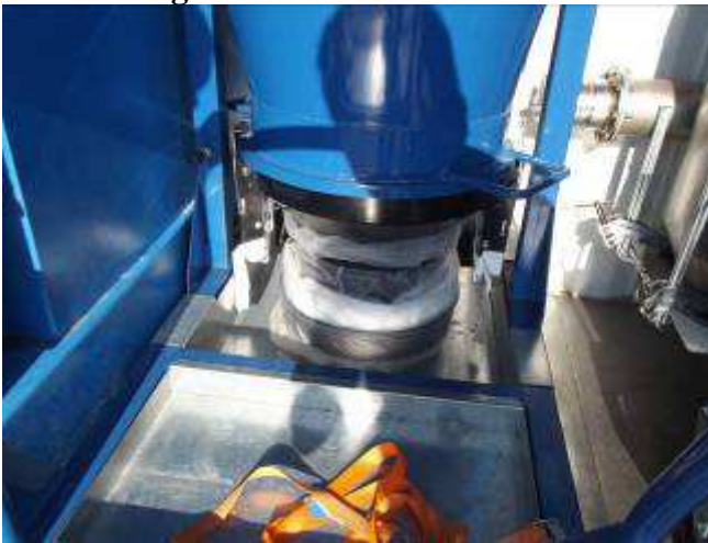
Recovery of UF 4 in Plastic Sacks
