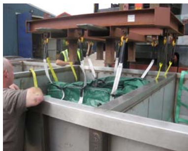
Figure 1 - SSP being lowered in to TC11 middle bay using the Lifting Frame
