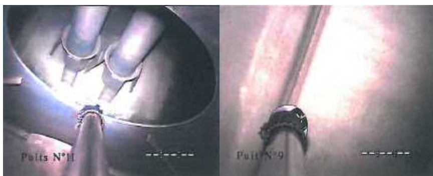
Figure 6: LR56 2004 corrosion inspection
