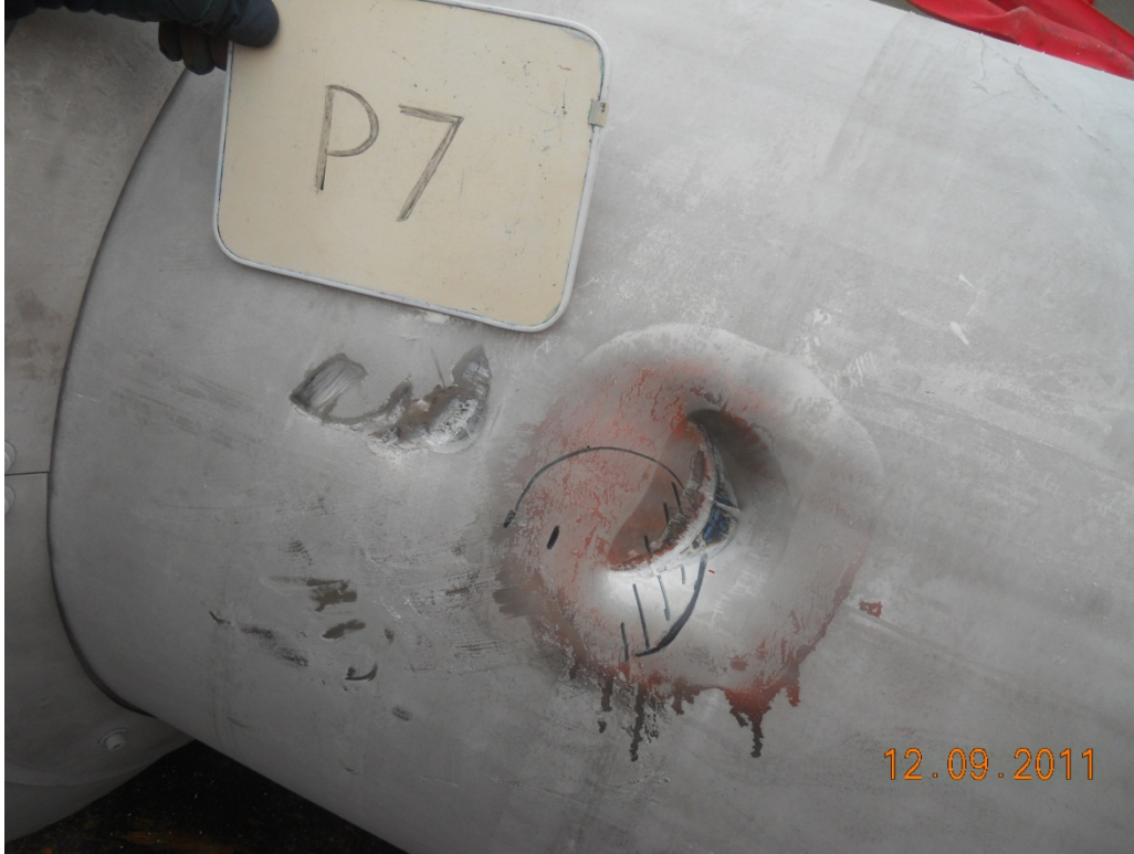
Figure 6. Puncture Damage to Thermal Shield
