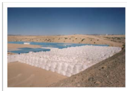
Stacked LiftPac's at NTS (Nevada Test Site, NV USA)
