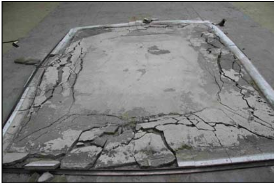
Figure 5. Destroyed mortar layer after drop test with DCI container
