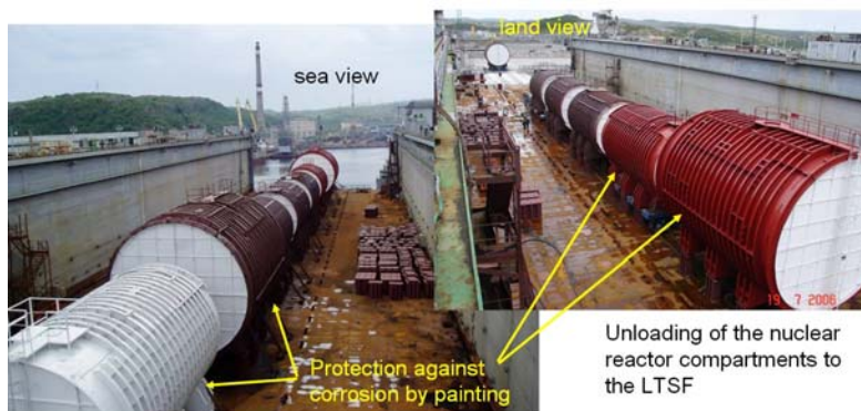
First transportation of 7 nuclear reactor compartments prepared for storage in the LTSF on the floating dock from the dockyard Nerpa to the Sayda Bay on July 2006
