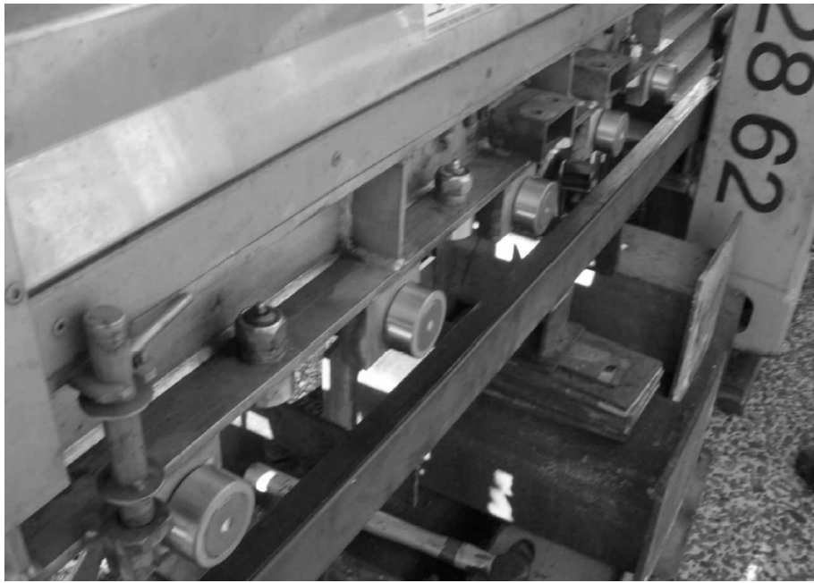
Photo 2. Roller of supporting frame
