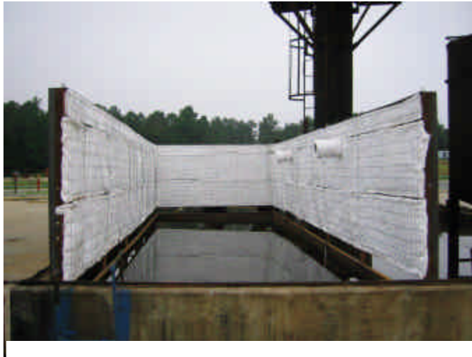
Figure 5 Insulated Interior of Burn Wall
