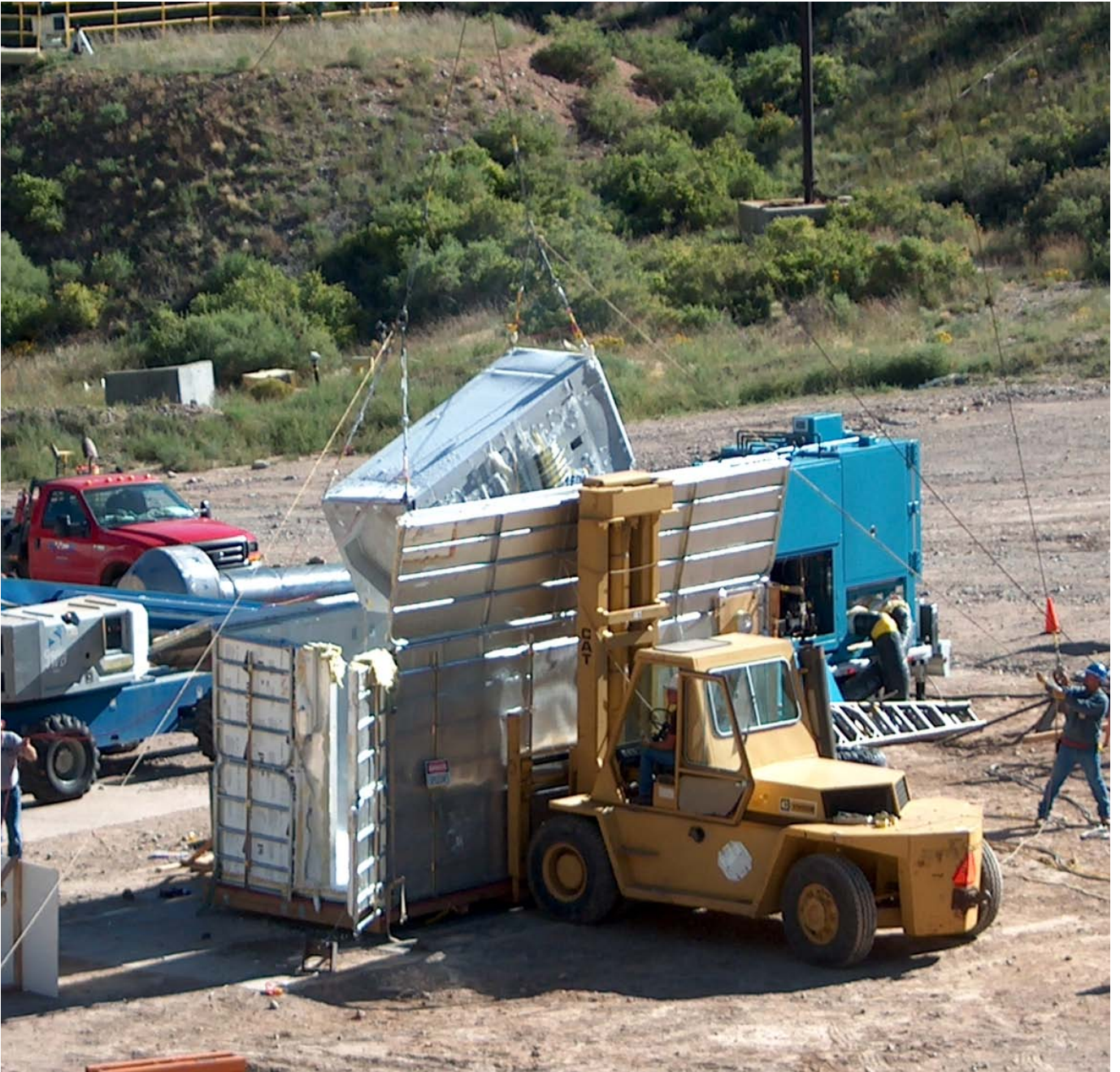
Figure 2 – Temporary Cooling Chamber. Portable Blast Chiller Unit is to the right of the open lid.
