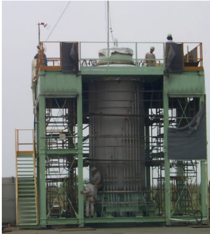
Figure5, Lead Pouring Equipment
