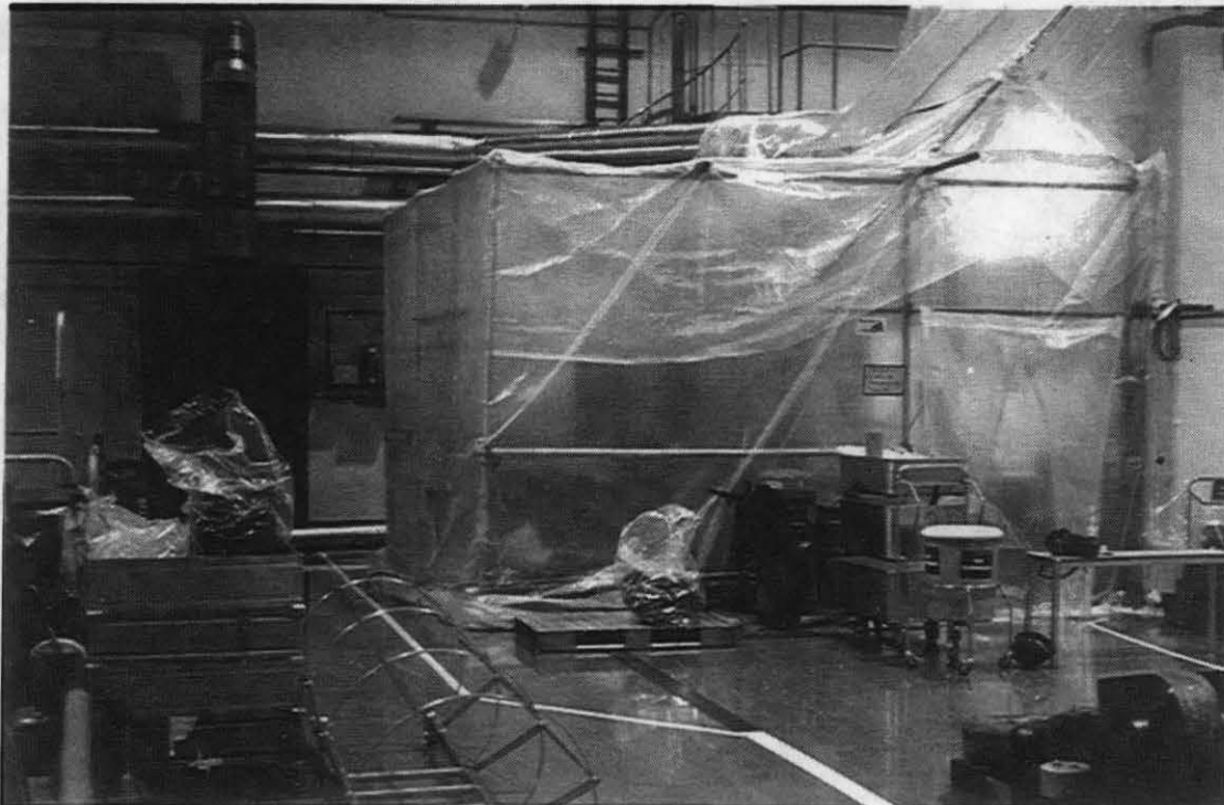
Temporary workshop at CLAB
