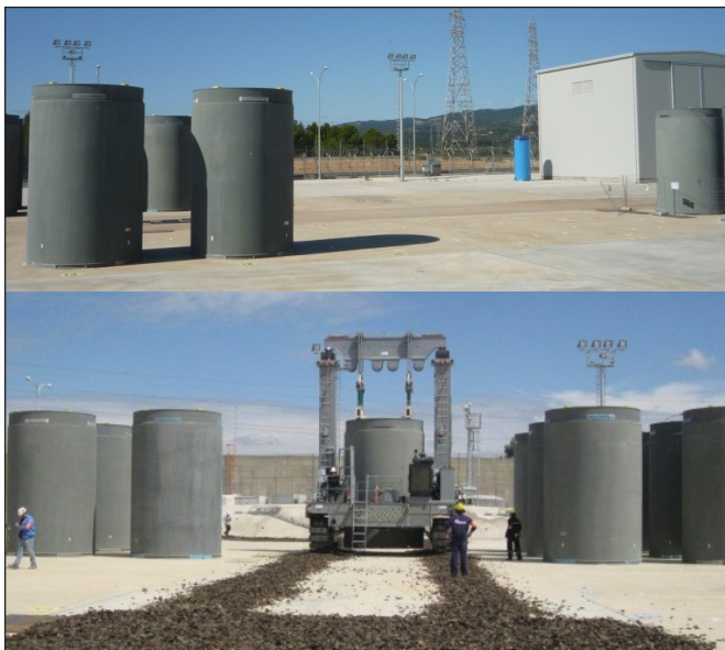
Figure 9. Ascó ISFSI and HI-STORM 100 in the concrete pad
