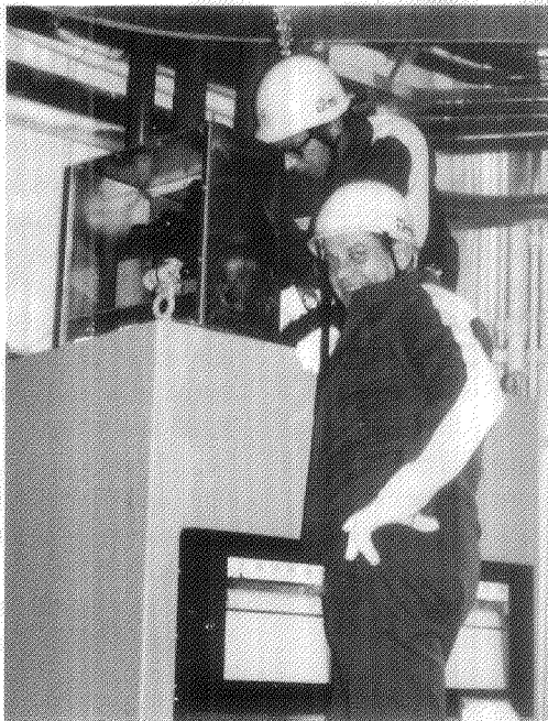
The author in 1971 installing a Contarex camera in one of the units of Tokyo Electric Power Co.'s Fukushima Dai-ichi Nuclear Power Station. Supervising from a lower level is safeguards veteran Cal Solem.
